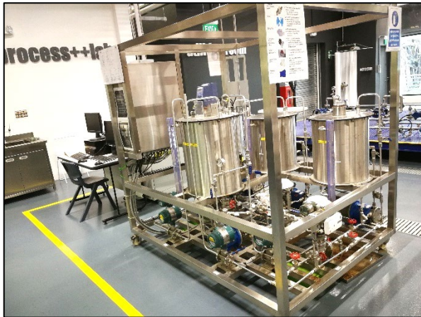
Figure 1. Actual Neutralizing Reactor Plant
